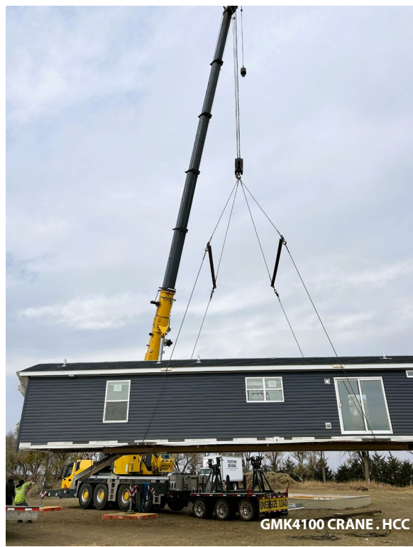
GMK4100 Crane HCC's new GMK4100 crane was used to set Western Housing homes for Tull Companies. Each half of a house weighed approximately 30,000 pounds.
