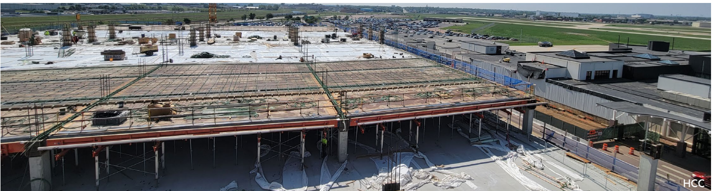
Sioux Falls Regional Airport Parking Ramp - Pictures from the Crane . Sioux Falls, SD 6 | HCC & ASCO & KCC
