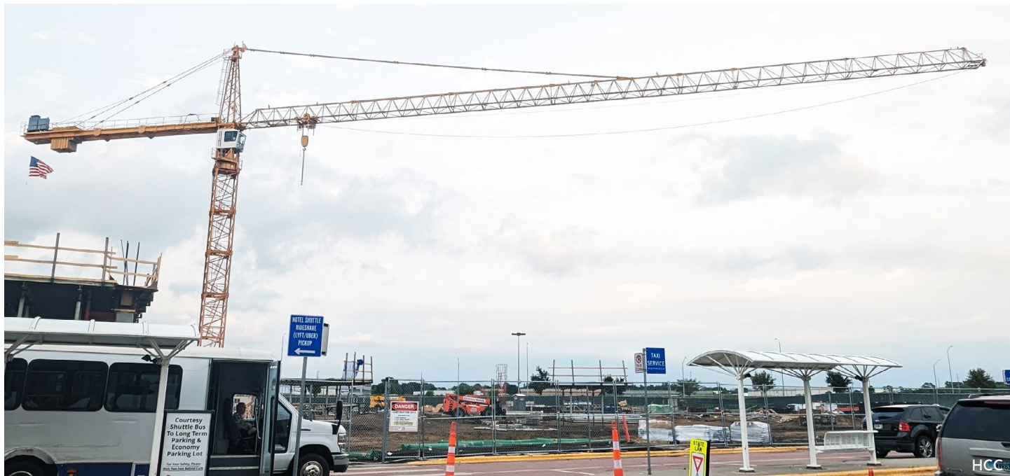
Sioux Falls Airport Parking Ramp Flags: Henry Carlson Construction crane operator and US Army veteran Todd Johnson volunteered to hang 8 foot by 12 foot American flags on the tower cranes at the Sioux Falls Regional Airport jobsite just in time for Independence Day. Thank you Todd!
